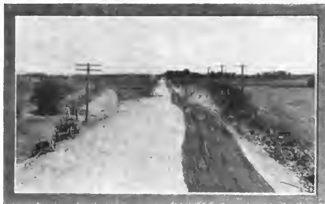
Showing how Britton's Hill has been cut down. Note the beginning of the oiling process on the right
